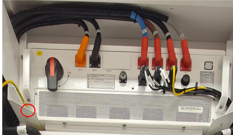
Figure 5-24 Position of Grounding Cable
