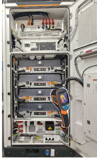
Figure 3-22 Measure with Thermal Imager
