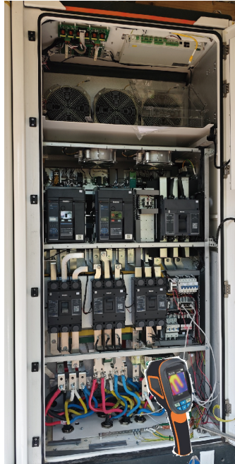
Figure 7-18 Measure with Thermal Imager
