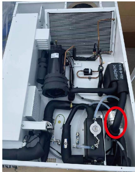
Figure 3-37 Pump of Liquid Cooling Unit
