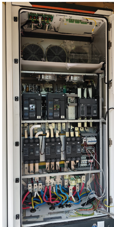
Figure 7-12 ATS Cabinet Interior
